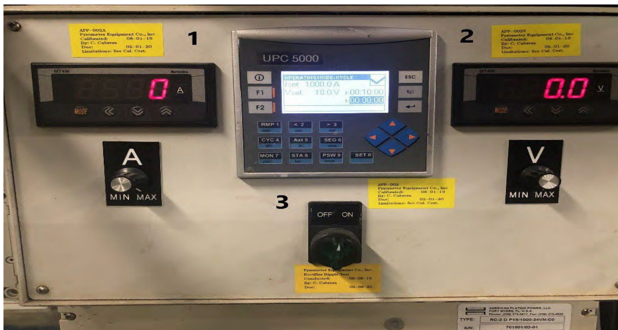
Figure 2.2 UPC 5000 computer module. (1) monitors the amperage on the system and (2) monitors the voltage on the system. To set the ramping process, the number of steps and current density levels were set in the touch screen (3).
