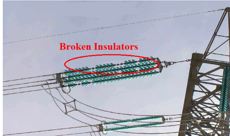
Figure 5.1: Missing faults in glass insulators of transmission lines.
