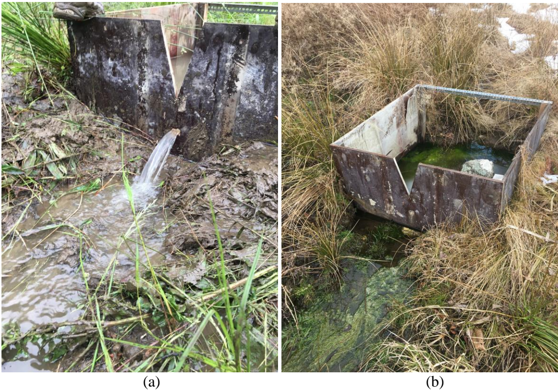
Figure 3.9 Orifice weir at outflows #1 during (a) Spring 2016 and (b) Winter 2017.
