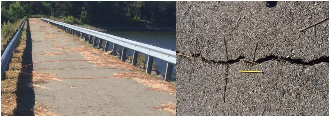
Figure 3.4 Transverse cracks along the crest.
