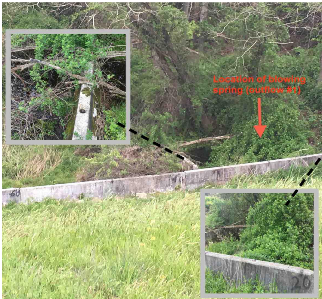
Figure 3.7 Location of blowing spring. Looking from the downstream slope towards the toe.
