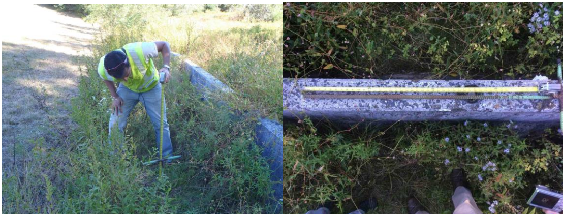
Figure 3.1 Detection of wet soft soil at the downstream toe.
