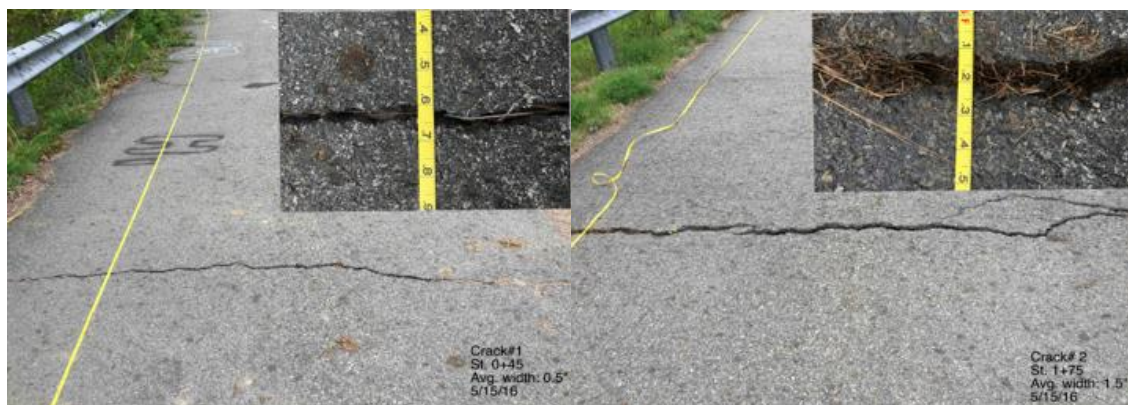
Figure 3.5 Location and status of observed transverse cracks along the crest (Continued).
