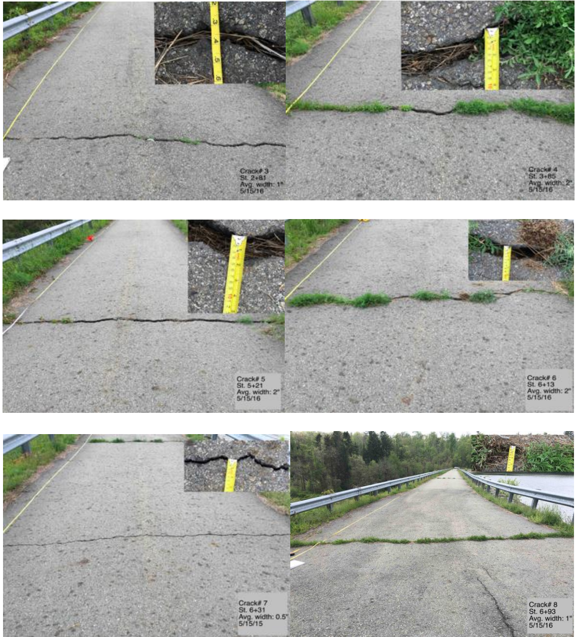
Figure 3.5 (Continued) Location and status of observed transverse cracks along the crest.
