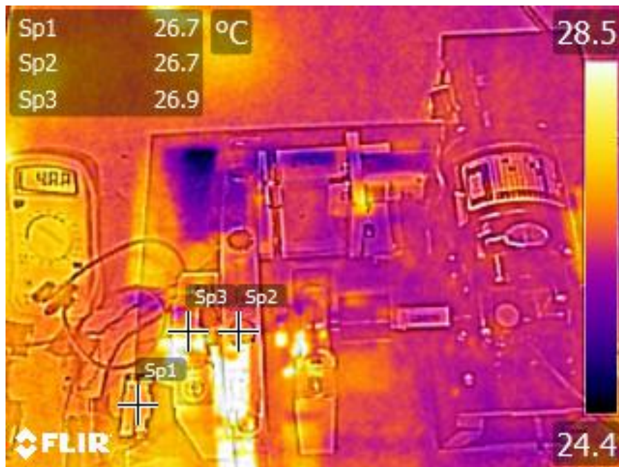
Figure 5.4 Thermal image of the charging system before charging.
