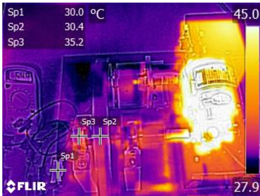
Figure 5.8 Thermal image of the charging system for charging for 40 minutes.
