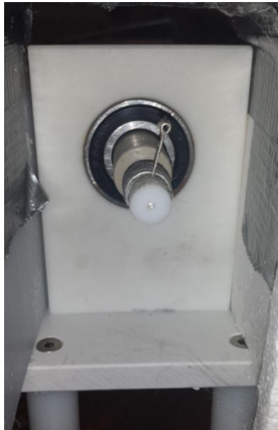
Figure 2.2 Picture of the slip ring with a protruding eye hook to allow for attachment of the grounding wire clip. This grounded eye hook is shielded by polyethylene housing.
