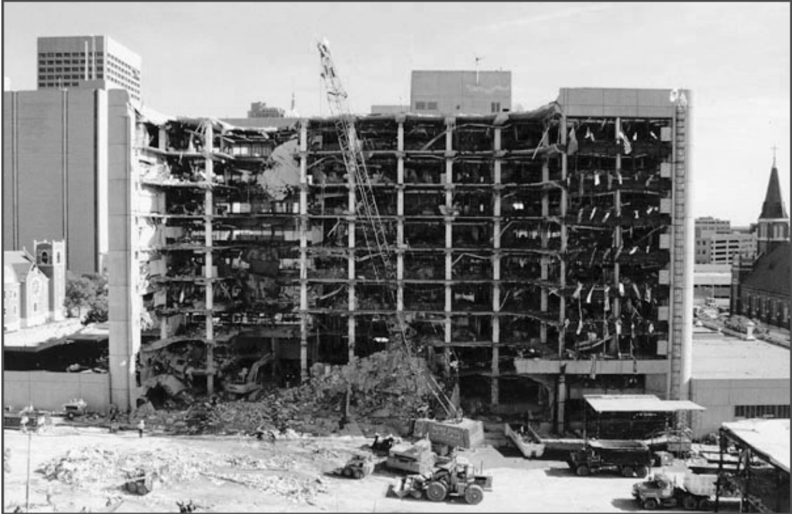
Figure 2.3 Exterior view of Alfred P. Murrah Federal Building after bombing and subsequent progressive collapse (FEMA 2003).
