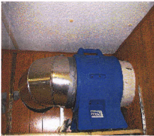
Figure 2.3 Fan to evacuate the fog.
