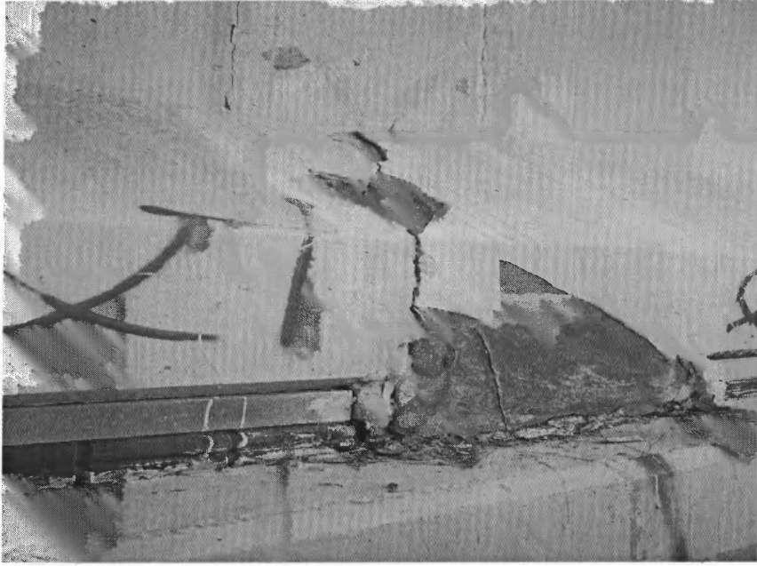
Figure 2.16 Diaphragm crack at fascia beam (Rt. 1&9, Newark).
