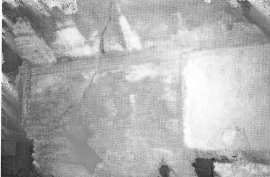
Figure 2.17 Typical diaphragm crack at inner beams (Rt. 1&9, Newark).
