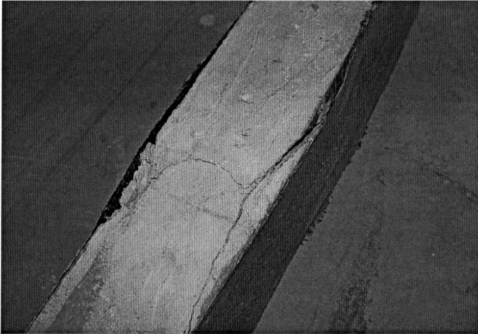
Figure 4.18 Failure of Beam Z31-FD.
