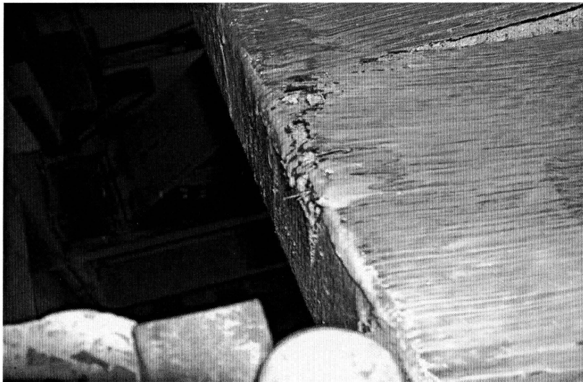
(b) Close-up view of the failure section
