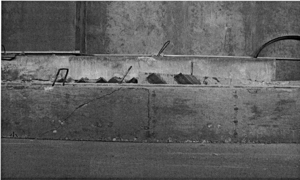
Figure 2.18 Failure of Beam ZC6(2).
