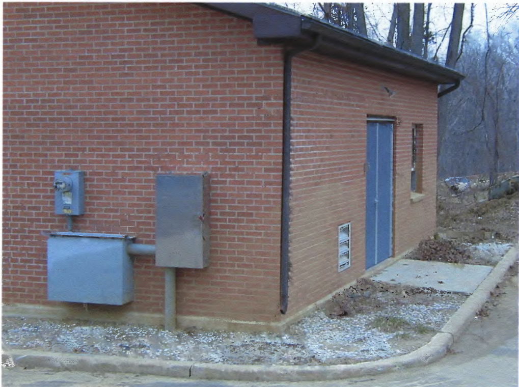
Figure 3.5 Photograph of Sparta pump house after partial clean up of landslide.
