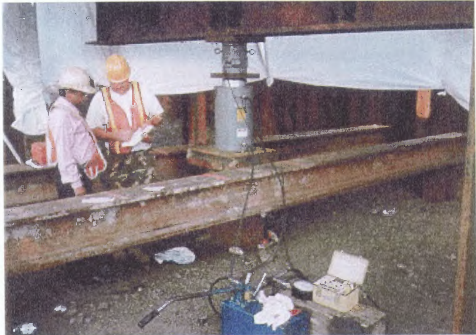
FIGURE B.8 Static Load Test Data Hydraulic Jack Assembly
