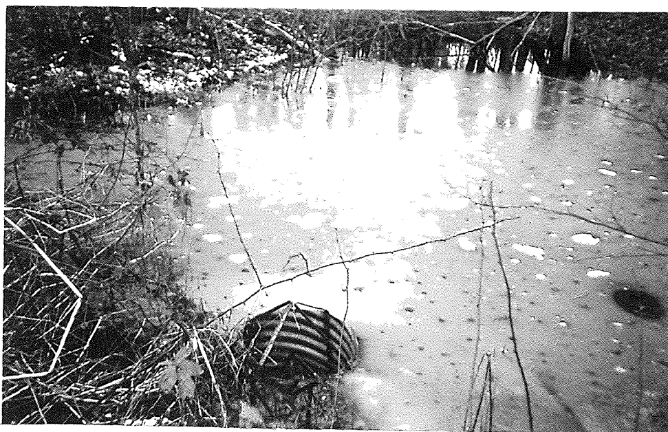
Figure 18 Photograph of Sediment Control Structure 4 retention basin as taken from Latonka Drive circumnavigating the Lake in Central Mercer County, Pennsylvania.
