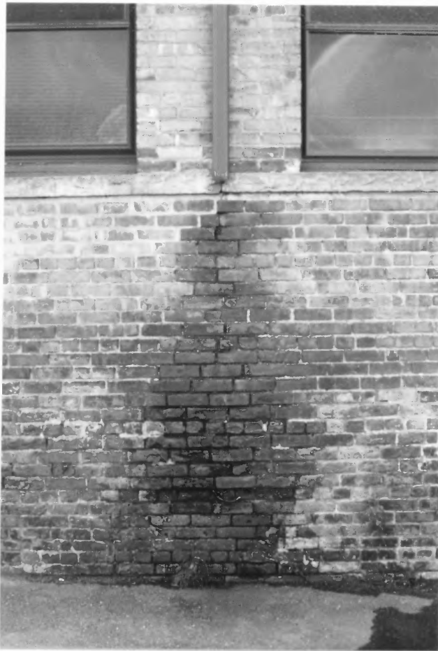
Fig.48. Wall washing caused by defective downspouts
